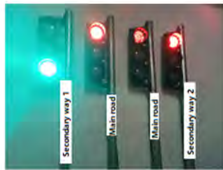
Figure 6. Activated state of lights on secondary way 1.
