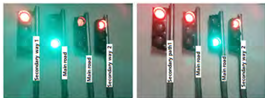
Figure 5. Active state of the lights on the main roads.
