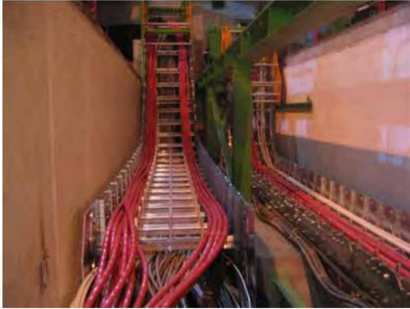
Figure 10.2: YB+2 and YE+1 cable-chains in UXC55 basement trenches.
