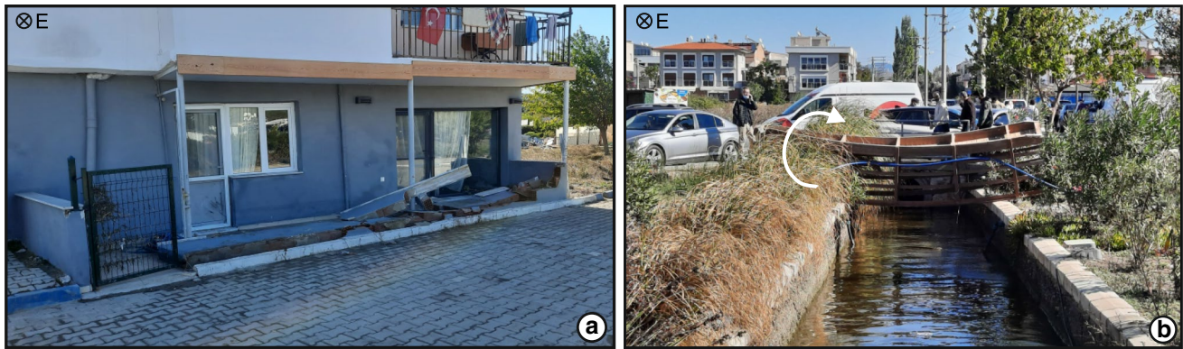
Fig. 7 a A 80-cm-high N–S-oriented wall facing the shore did not resist the tsunami destroyed walls. b A bridge on the E–W was drifted and toppled by the waves
